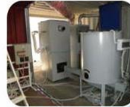
Feeding system and heat exchanger
